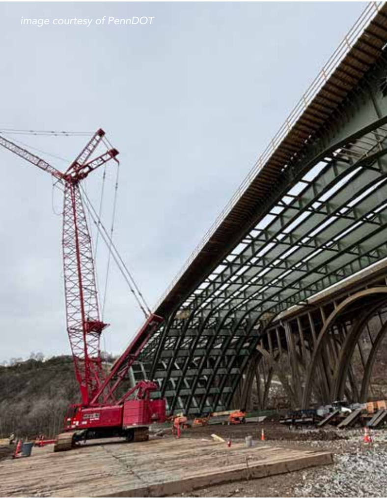
A bridge slide-in outside the Squirrel Hill Tunnel image courtesy of PennDOT
