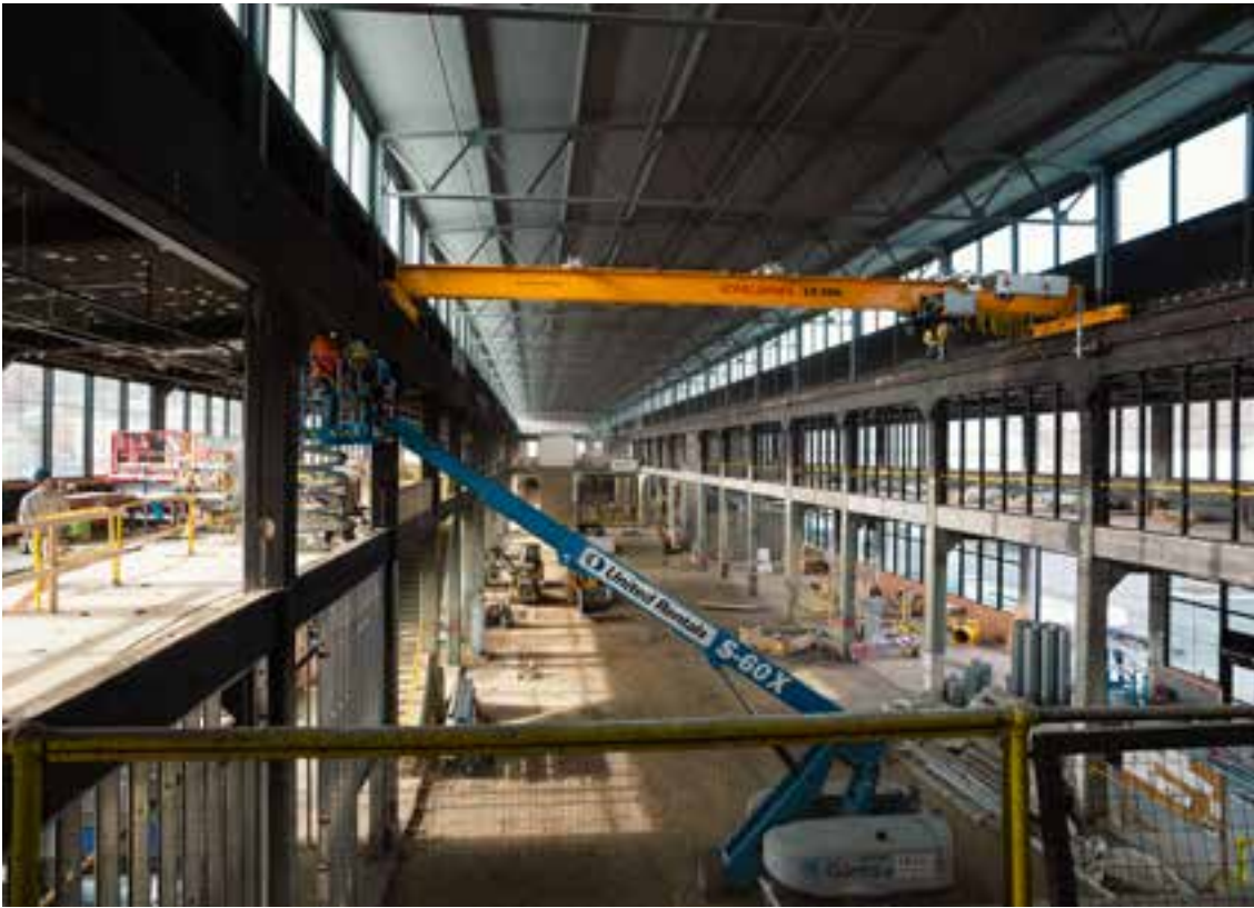
The massive high-bay space will be used as a maker space/manufacturing facility. Photo by 80HD Media House.
